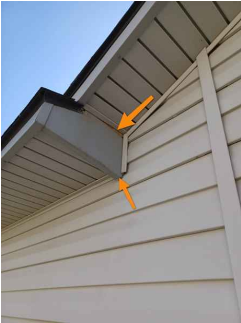
Fascia has slipped down
