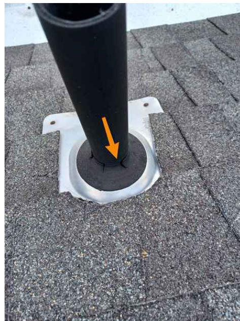
Cracked weather boot
