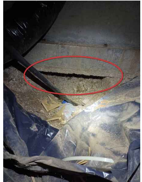
Approximately 3 feet of the concrete foundation has been dug out and left unsupported
