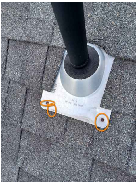
Exposed nail heads in flashing
