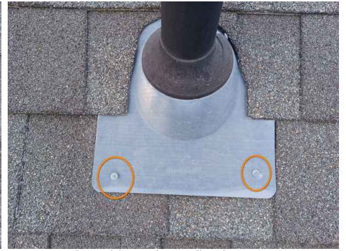
Exposed nail heads in flashing
