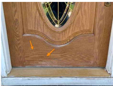
Front door damage at the bottom
