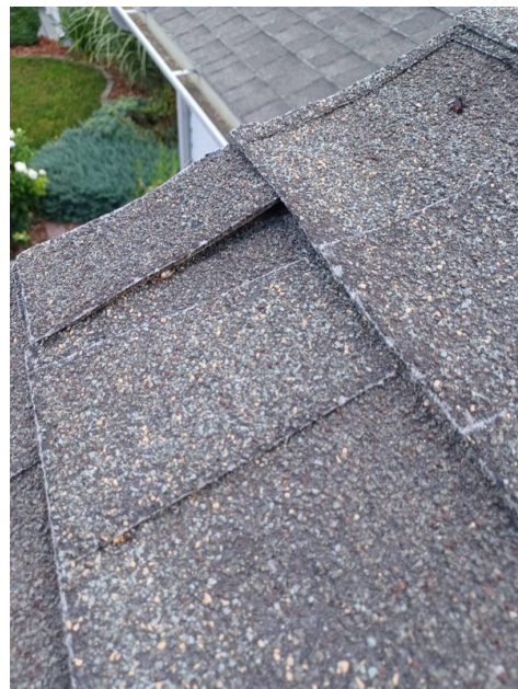
Granular loss along edges of shingles exposing fiberglass layer
