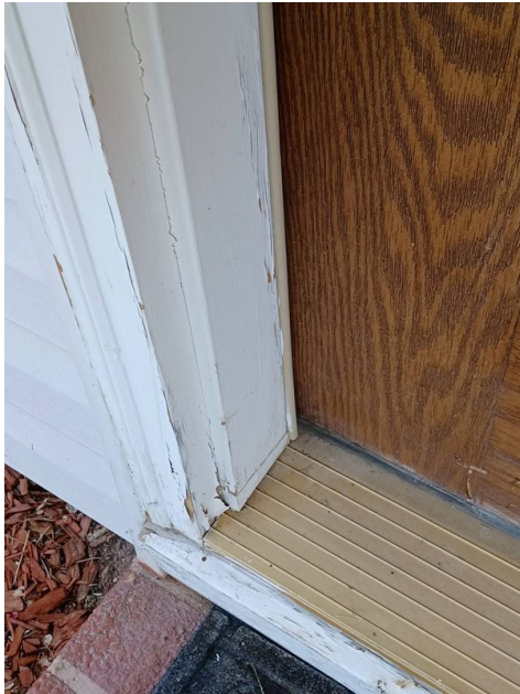
Front door trim damage
