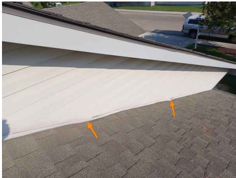
Warped siding and trim piece. Trim piece has separated.
