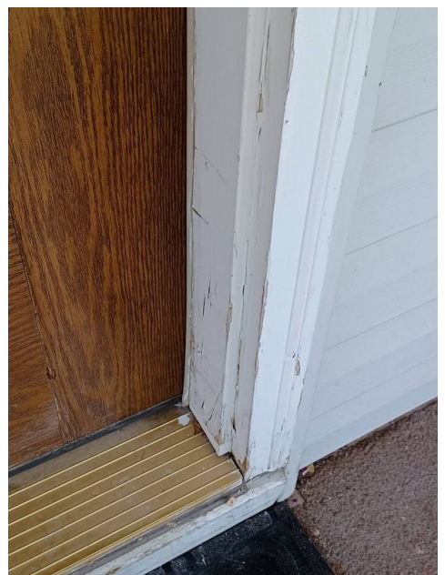
Front door room damage
