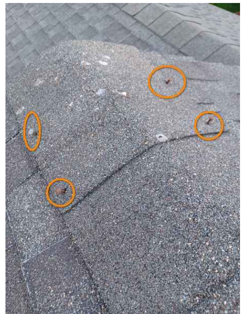
Under driven nails on the ridge
