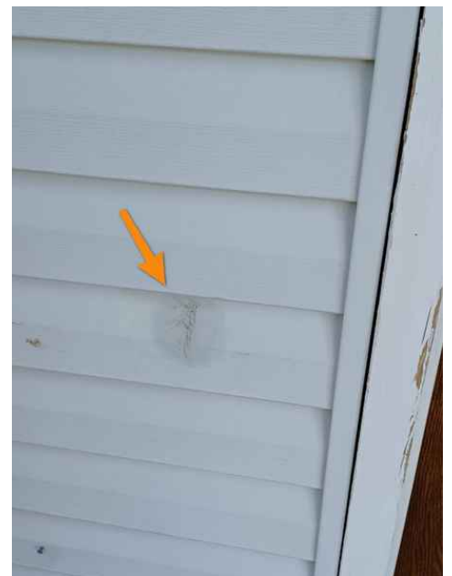
Siding crack near the front door
