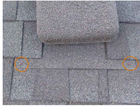
Exposed nail heads in flashing
