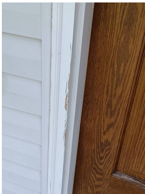
Front door trim damage
