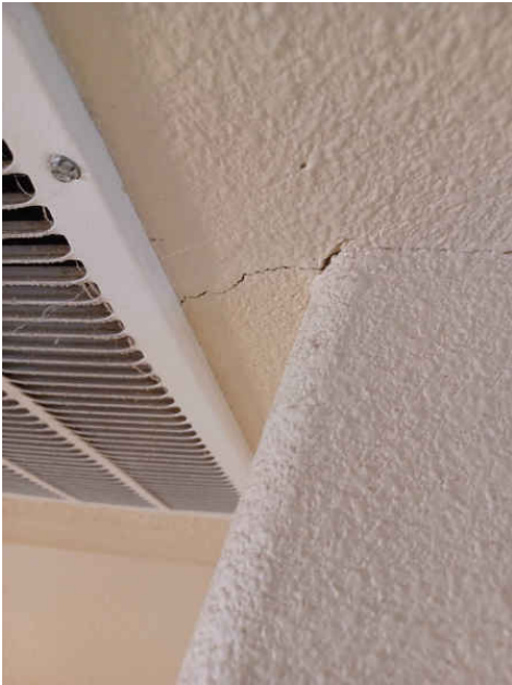
Crack in the drywall at the forced air return
