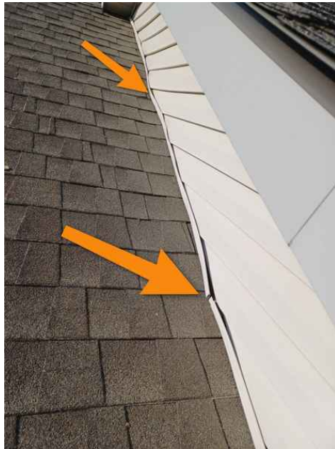
Warped siding and separated trim piece
