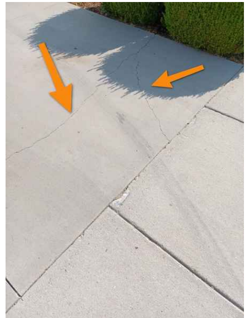
Cracks on the driveway
