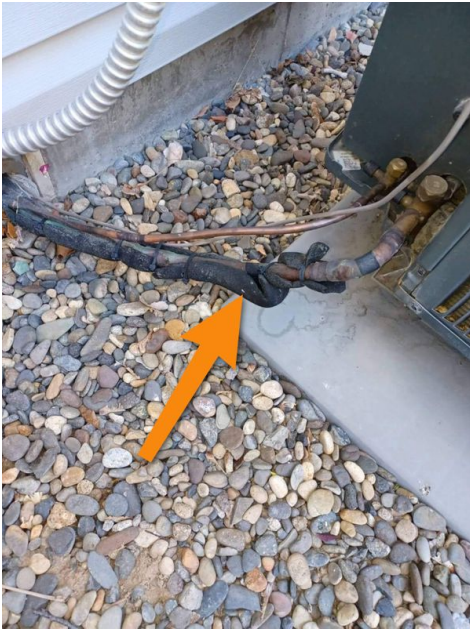
Incomplete insulation on refrigerant lines
