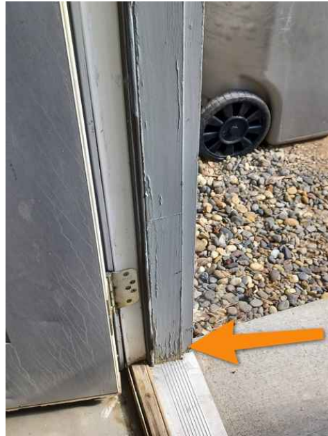
Man-door from garage trim damage
