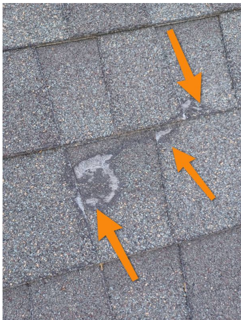
Complete loss of granules revealing fiberglass layer
