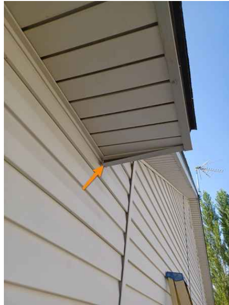
Fascia has slipped down
