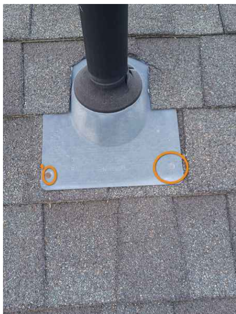
Exposed nail head in flashing
