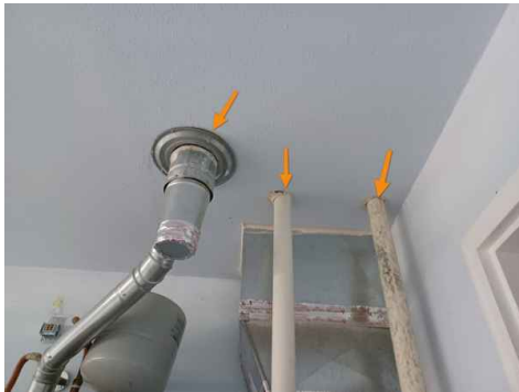
Cracked and missing caulking
