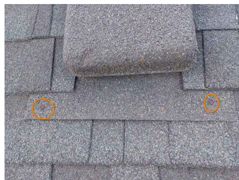
Exposed nail heads in flashing
