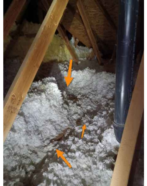
Insulation has settled or been moved in areas of the attic.
