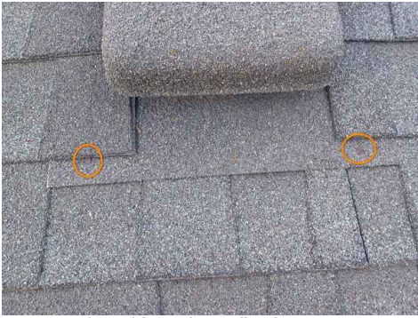
Exposed nail heads in flashing
