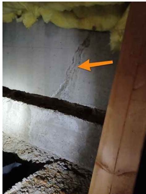
Efflorescence at small crack in the concrete foundation
