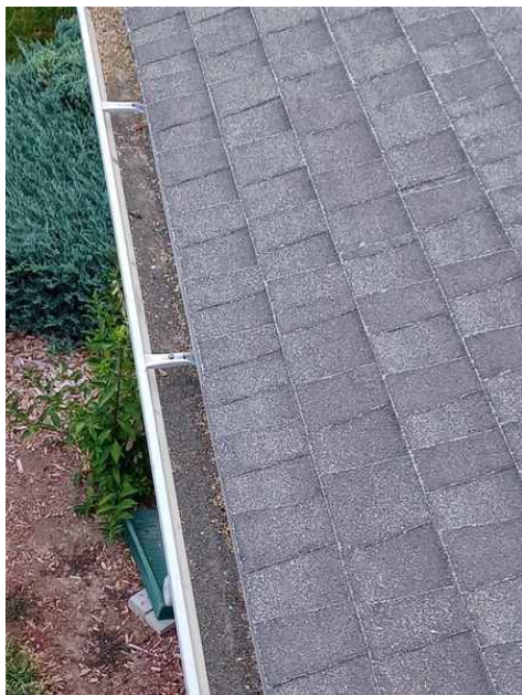
Dirt and debris accumulation in gutter
