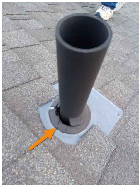
Damaged weather boot
