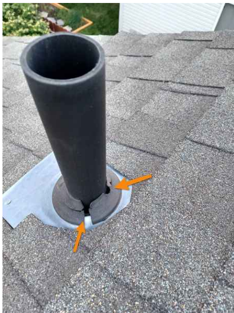
Damaged weather boot
