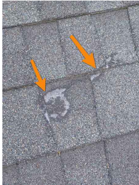
Shingle worn through. Granules and asphalt layer of shingle worn away exposing the fiberglass layer
