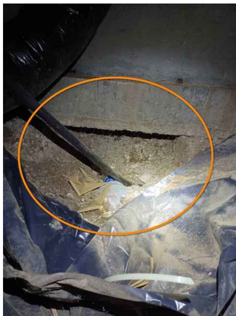
Vapor retarder pulled back exposing dirt
