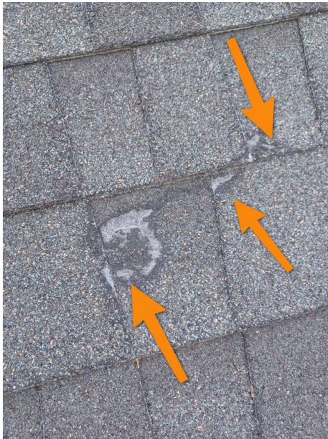
Complete loss of granules revealing fiberglass layer
