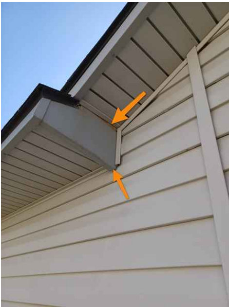
Fascia has slipped down
