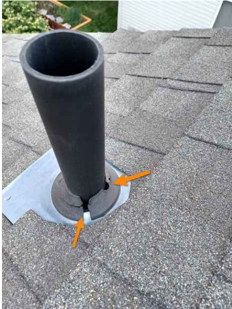
Damaged weather boot
