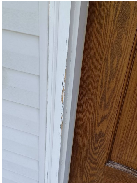
Front door trim damage
