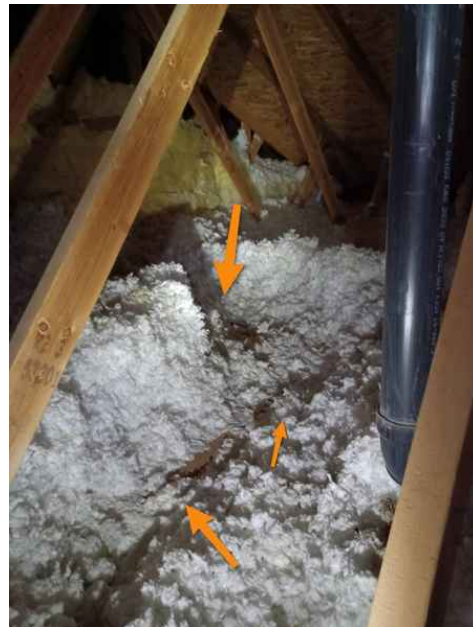
Insulation has settled or been moved in areas of the attic.
