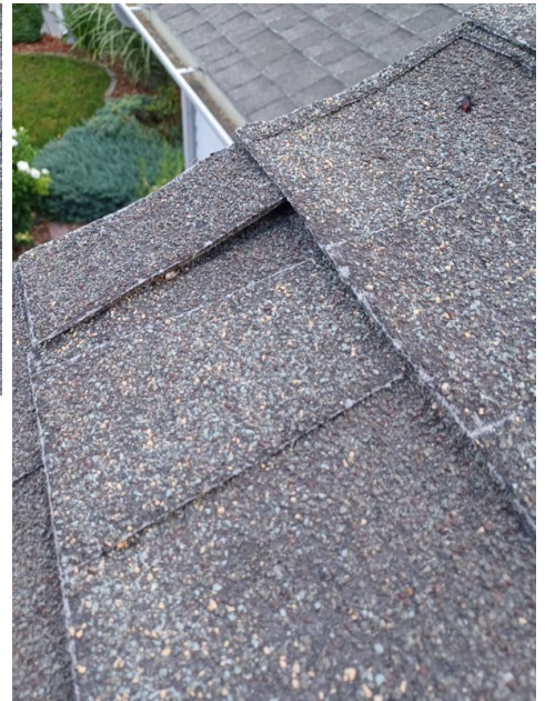
Granular loss along edges of shingles exposing fiberglass layer
