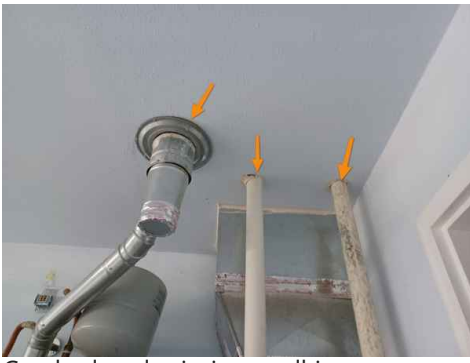
Cracked and missing caulking
