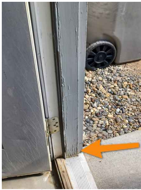
Man-door from garage trim damage
