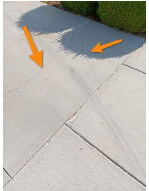
Cracks on the driveway
