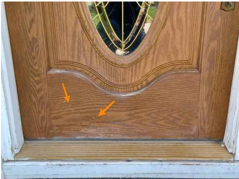
Front door damage at the bottom
