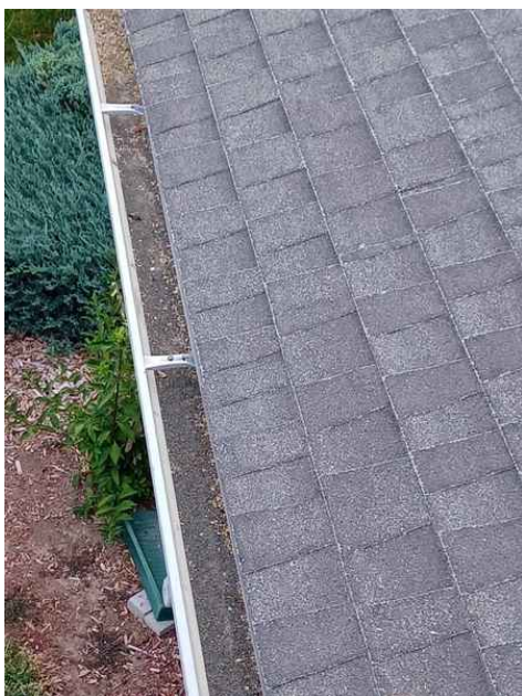
Dirt and debris accumulation in gutter
