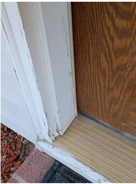
Front door trim damage
