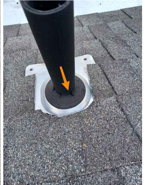
Cracked weather boot
