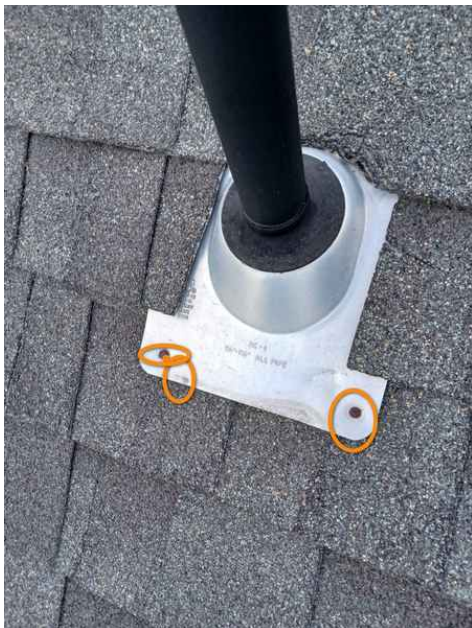
Exposed nail heads in flashing
