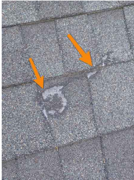
Shingle worn through. Granules and asphalt layer of shingle worn away exposing the fiberglass layer
