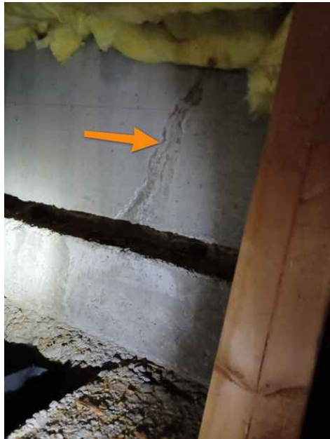
Small crack at west side of foundation wall
