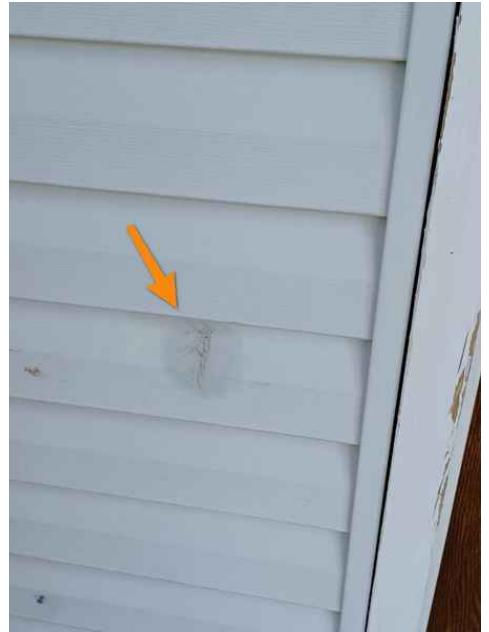
Siding crack near the front door
