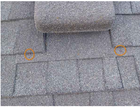
Exposed nail heads in flashing
