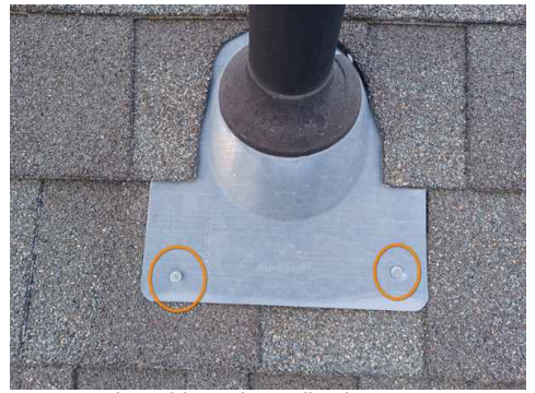
Exposed nail heads in flashing
