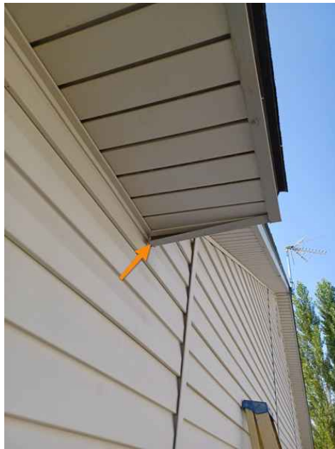
Fascia has slipped down
