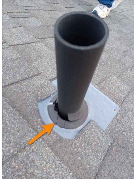
Damaged weather boot
