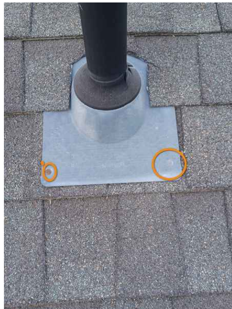
Exposed nail head in flashing
