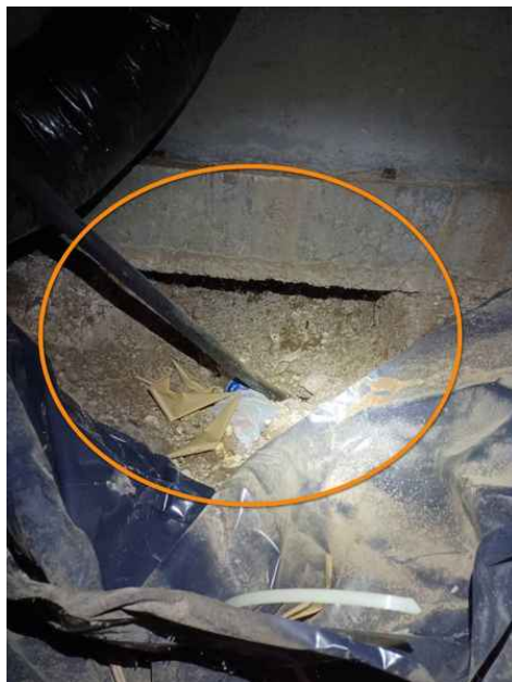
Vapor retarder pulled back exposing dirt
