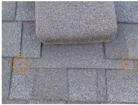
Exposed nail heads in flashing
