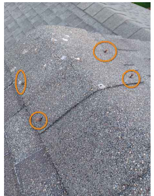
Under driven nails on the ridge
