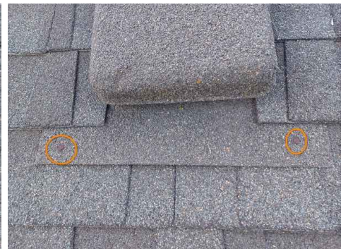
Exposed nail heads in flashing
