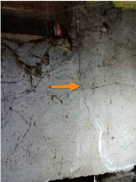
Small crack at west side of home's foundation
