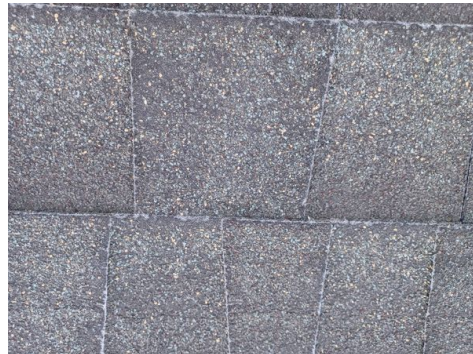
Fiberglass visible along edges of the shingles
