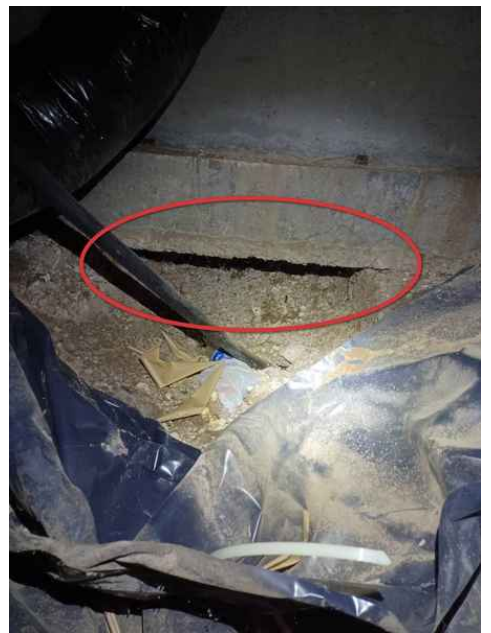
Approximately 3 feet of the concrete foundation has been dug out and left unsupported
